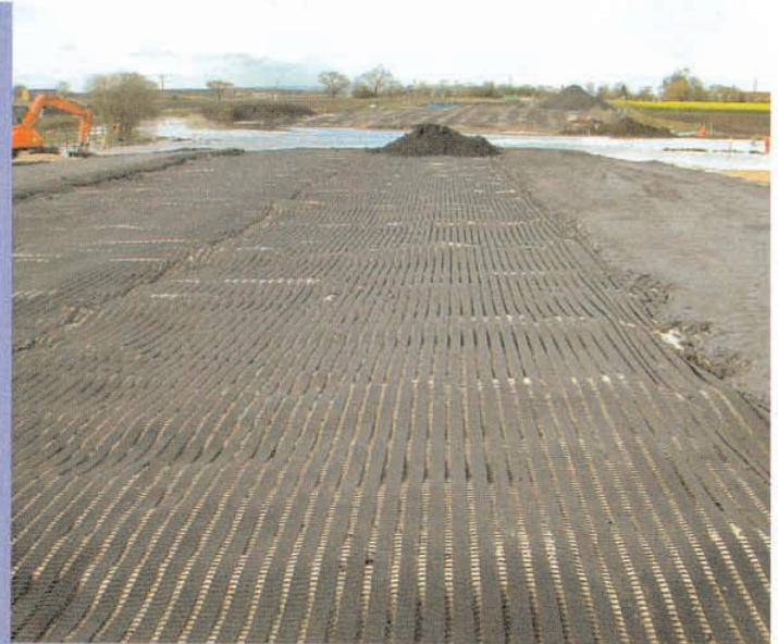
A change in pile layout allowed the same grade of geosynthetic to be used in both directions on the embankment.
