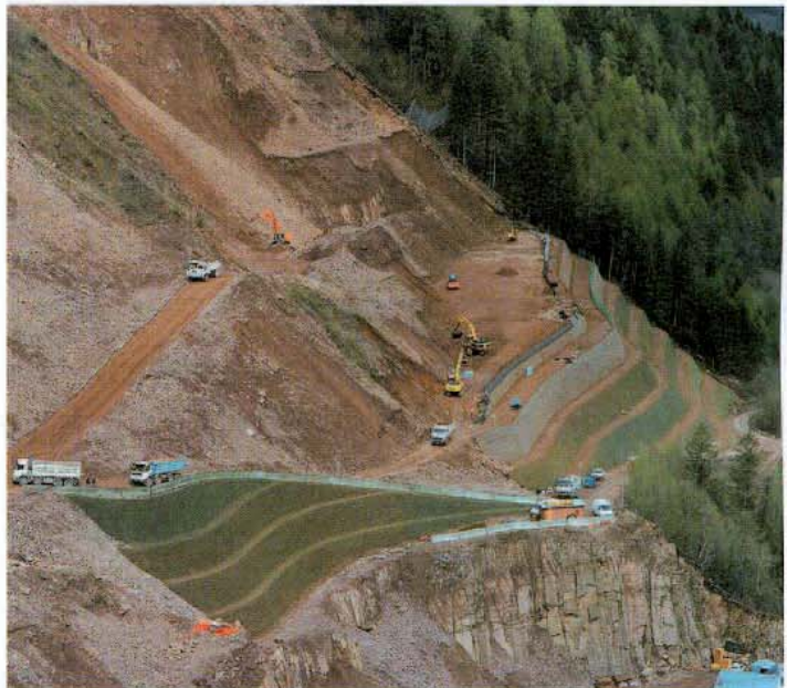
The 60m high slope at Lases has been benched and reinforced with geotextile to prevent a potentially catastrophic failure.
