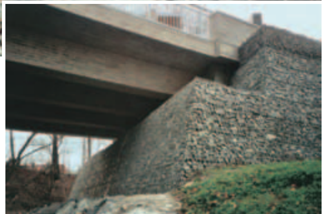
Load transfer takes place through the GRS structure onto which the abutment bearing shelf is directly cast.
