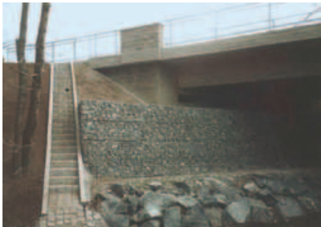
The facing is constructed from galvanised gabion cages filled with crushed stone / armour stone.
